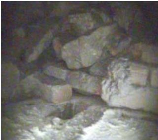
The above borehole camera stills show the lining/rock interface and void over lining in a rail tunnel.
