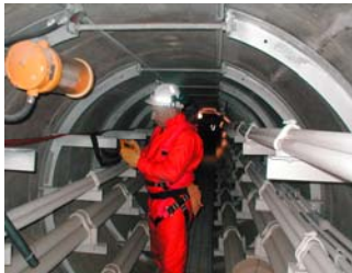
Reading instrumentation installed in one of the CTRL Tunnels
